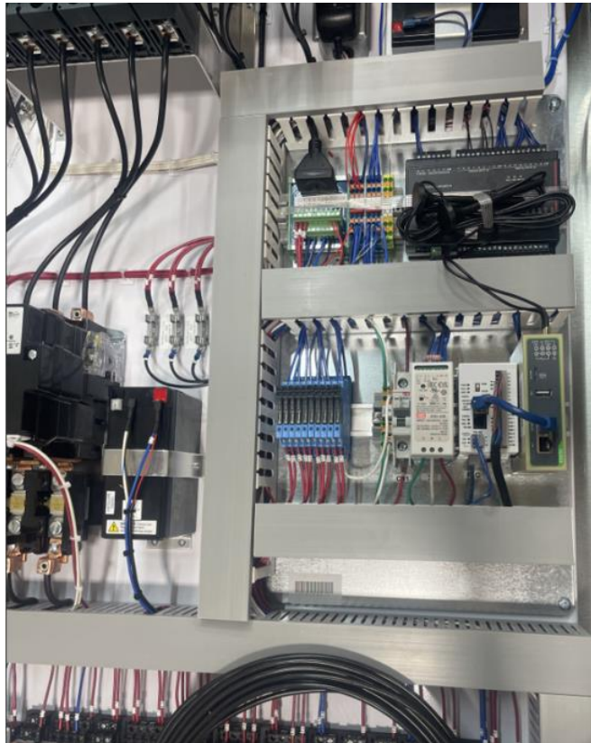
Example of a Mounted STREAMETRIC Unit with No Enclosure Inside a Station's Main Control Panel
